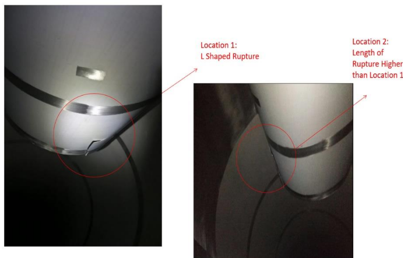
Figure 1: Crack on cyclone insert cone.
