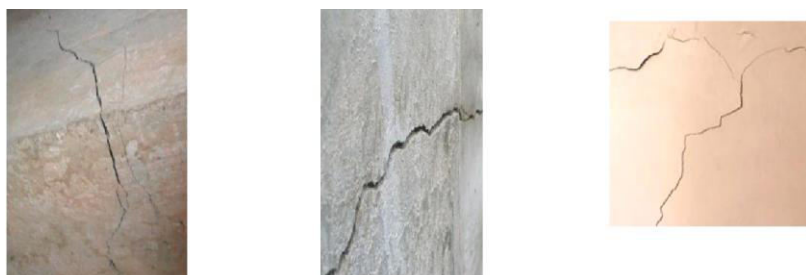
Figure 1: Cracks in building structures:(a)concrete wall,(b)concrete beam and(c)brick wall with mortar surface
