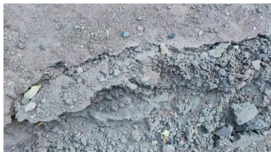
Figure – Edge Cracking
