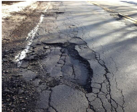
Figure – Longitudinal cracking
