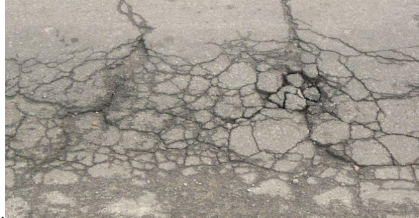
Figure – Block cracking
