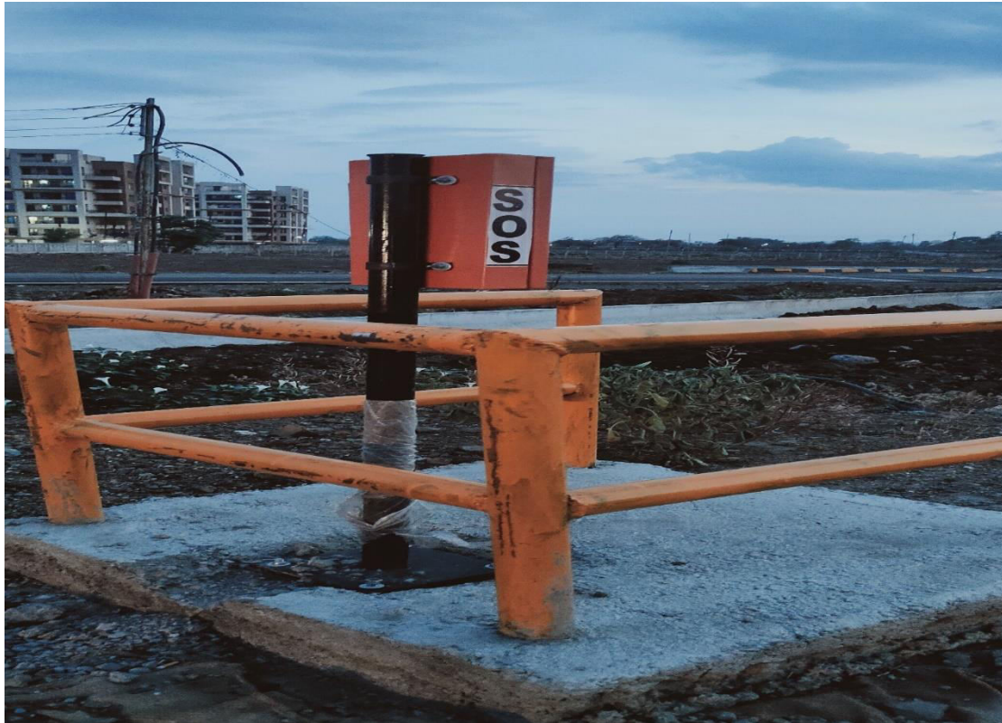
Fig 13: Emergency Roadside Telephone System At Nagpur-Umred Road
