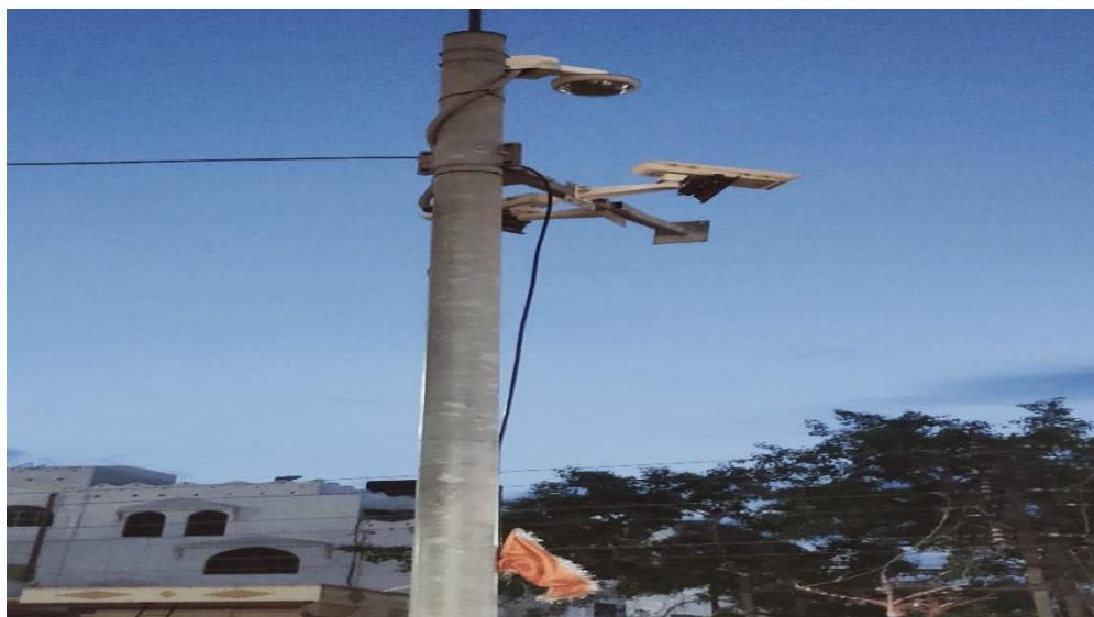
Fig 10:- Video Surveillance System CCTV
