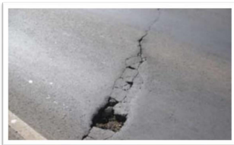
Fig 2: Potholes on Kalmeshwar Road
